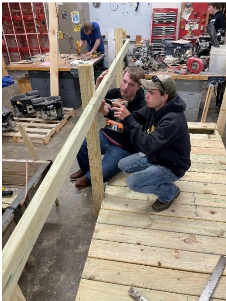
The Tech Ed department helped a local couple to build their own ramp for wheelchair accessibility. Pictured, seniors attach the handrail to the ramp.
